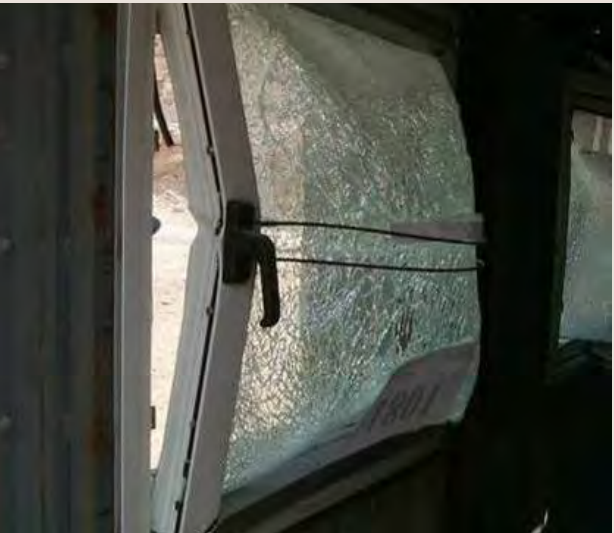
Figure 42: Window after explosion
